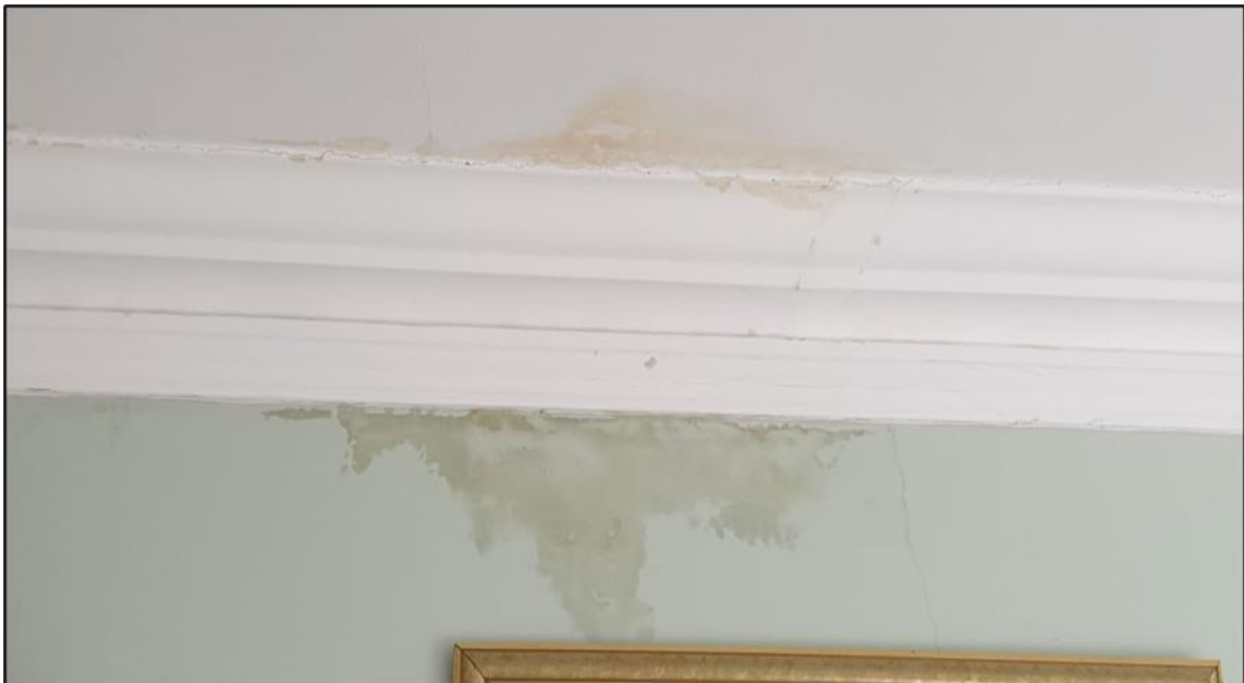
Figure 7: Water damage at 2F, 10 Randolph Crescent due to leaking roof.
